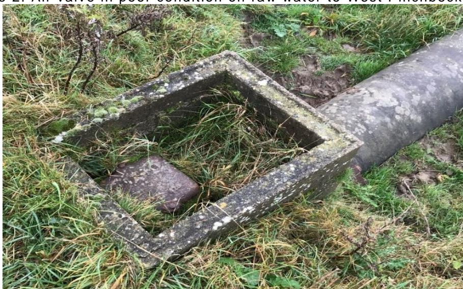
Figure 2: Air valve in poor condition on raw water to West Pinchbeck works
